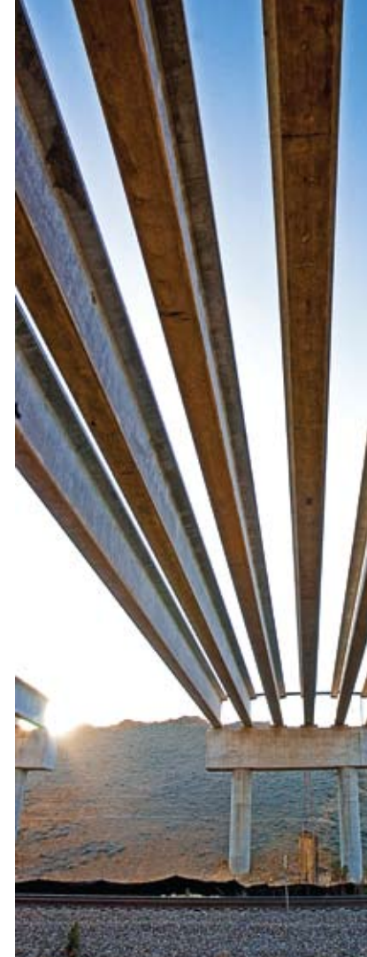
Construction of the ALDOT overpass at the intersection of US Highway 43 and ThyssenKrupp Drive continues to progress. The overpass will provide access to trucks entering and exiting the ThyssenKrupp Steel USA facility.
