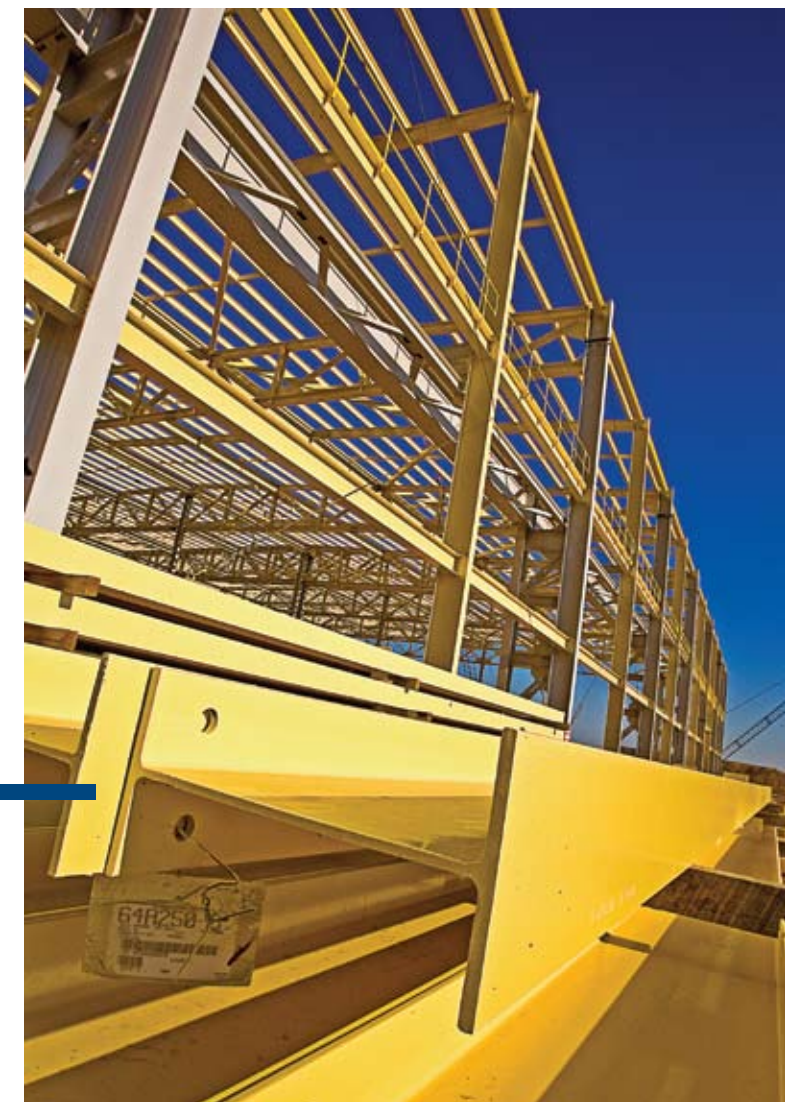
Above, ThyssenKrupp Steel USA will make use of the ThyssenKrupp “Pilot Line” for development of improved surface coatings. Right, steel erection has already begun in the Cold Rolling Mill’s storage area.
