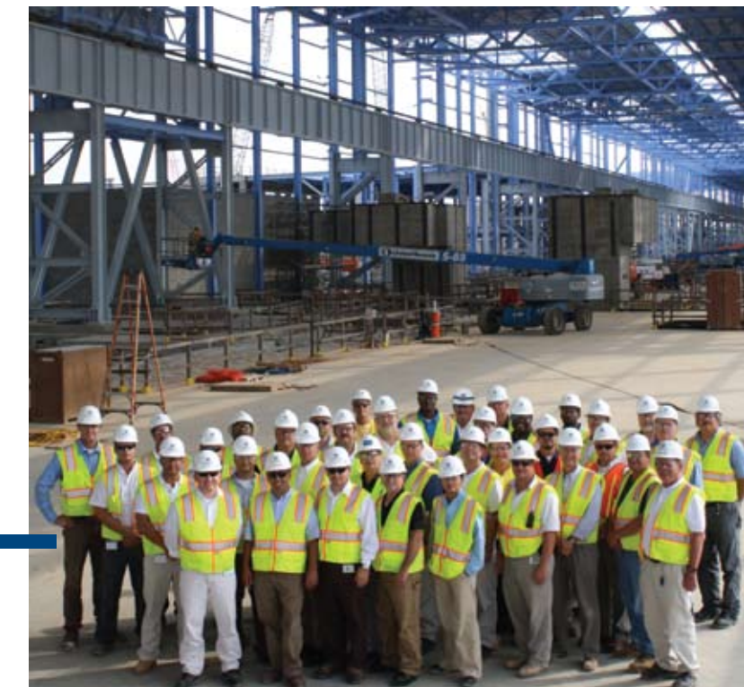
ThyssenKrupp Steel USA's hot strip mill team in the furnace area of the mill currently under construction. The mill will have three walking-beam furnaces, two roughing mill stands and seven finishing mill stands ready to coil 16 gauge product all the way up to 1" in thickness.
