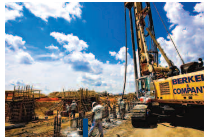
Construction of ThyssenKrupp Steel USA's carbon steel processing facility is going vertical as completion of piling and foundation work approaches
