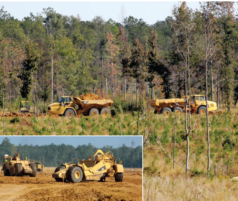
Hundreds of specialized heavy equipment vehicles have been working to prepare the new site for construction in Calvert, Alabama, since the May 2007 announcement.
